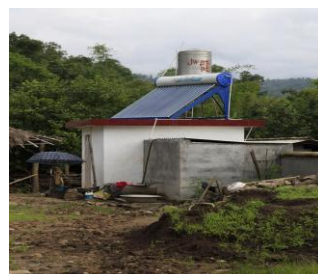
The best toilet facility (not requiring inclusion in the project) with a solar-powered water heater on the roof.
