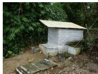
A toilet connected to a methane pit built with brick walls, cement floor and iron roof.
